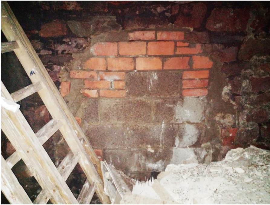
The bricked-up entrance to the horizontal flue can be seen on the west wall of the boiler house
